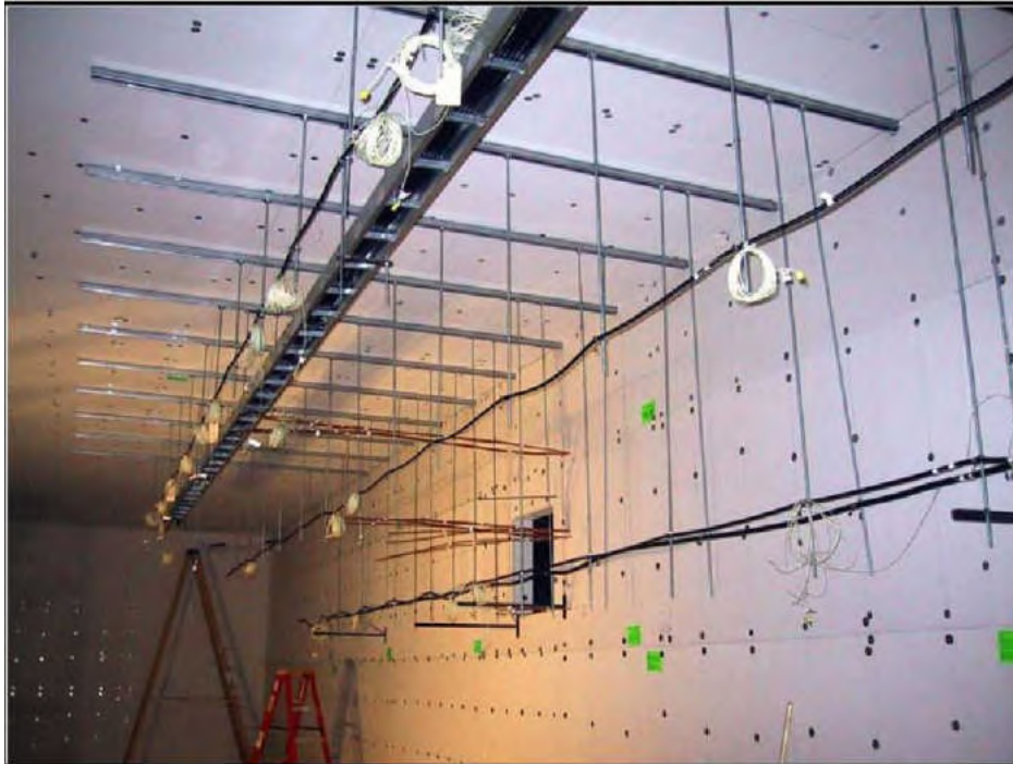
Figure 2-5 Cables in Compartment for Benchmark Exercise No. 3
